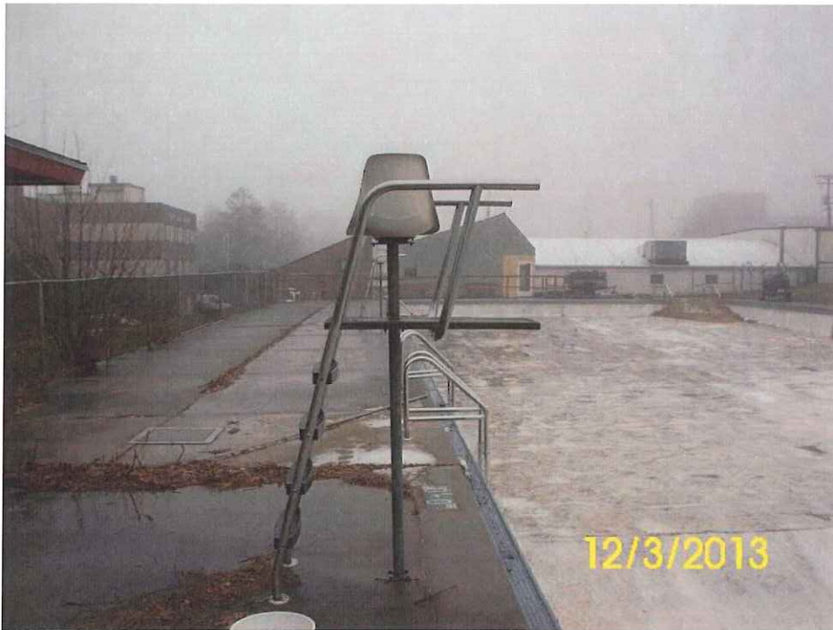
Decking – West Side, Repair and Partial Replacement Required
