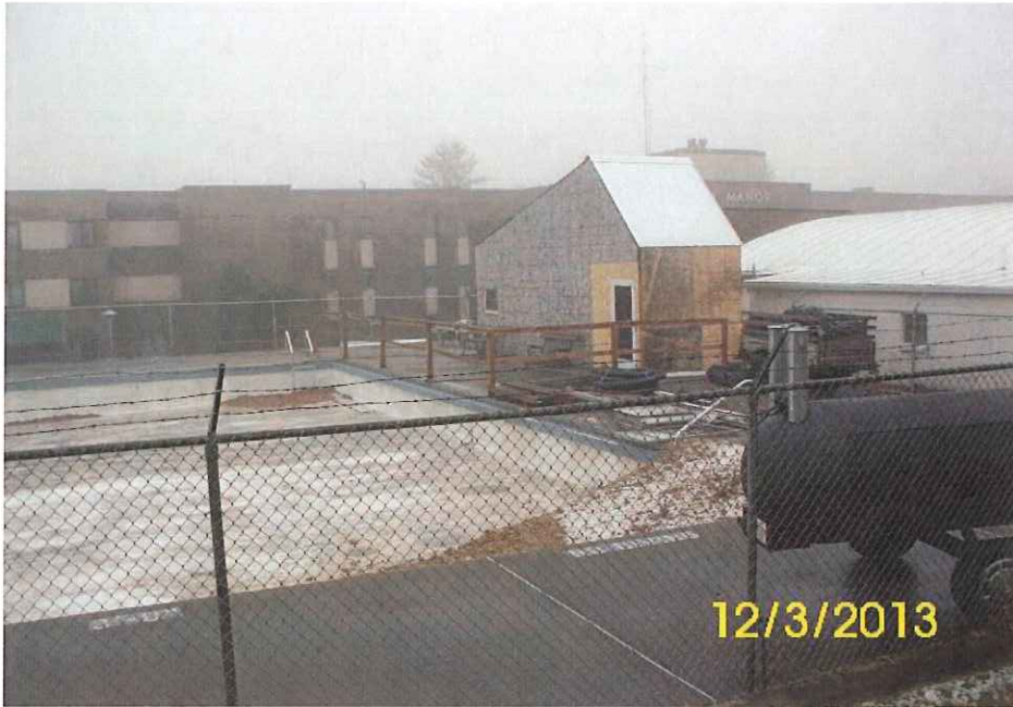
Deck – North Side, Partial to complete replacement required
