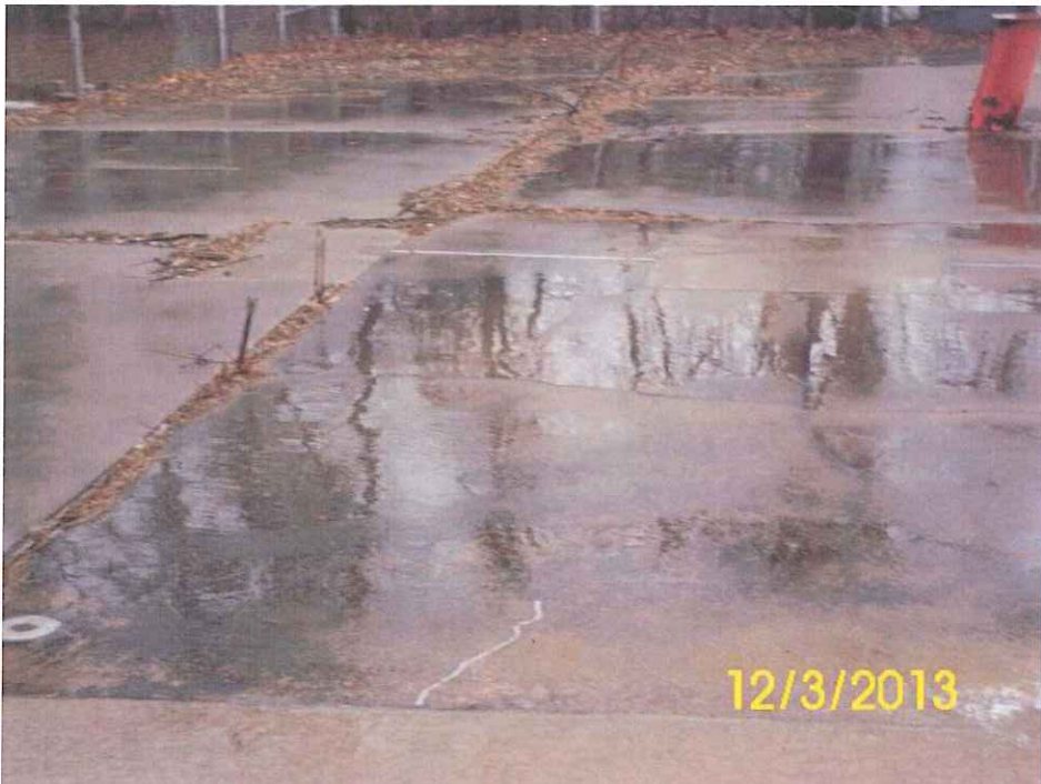
Deck – South Side, Complete Replacement Require
