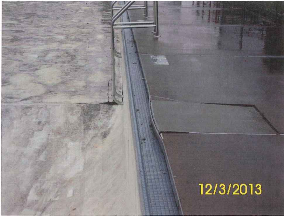
Deck – East Side, Partial Replacement Required
