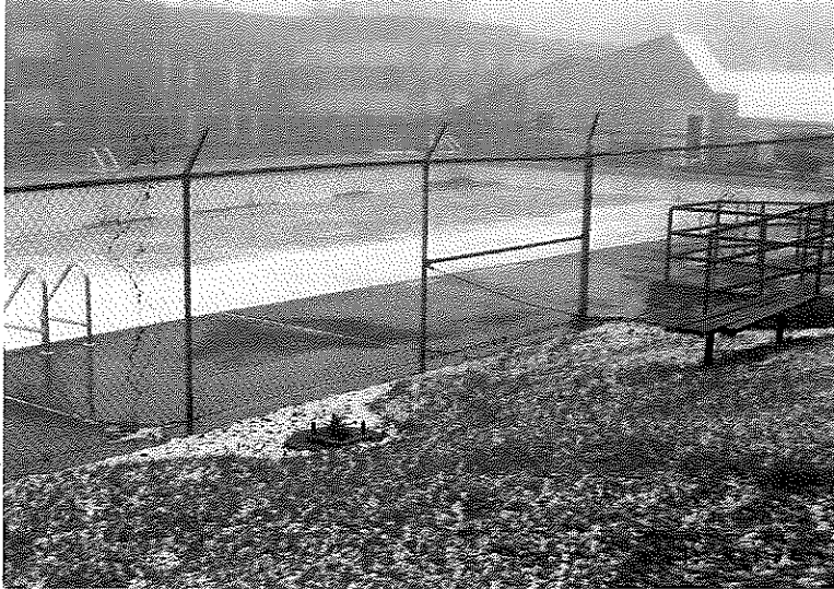
Typical light pole base
