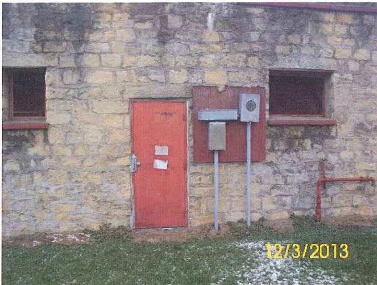
Bathroom Doors – Poor condition, Hardware not ADA
