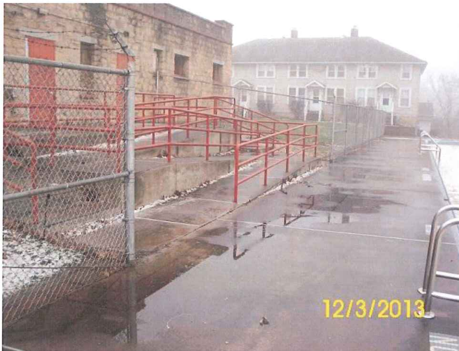
Ramp to bathhouse, note lack of deck drain
