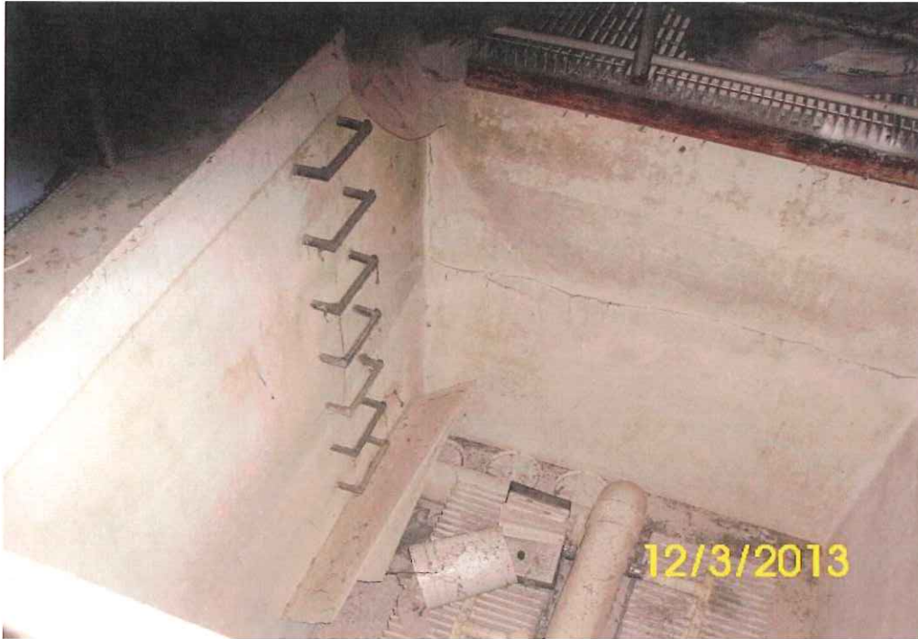
Surge Tank/Filter Tank
