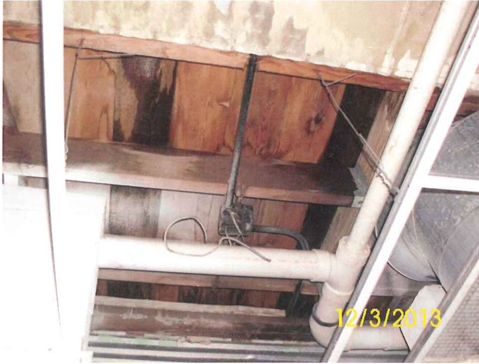
Wood Rafter Structure – Wet and rotting
